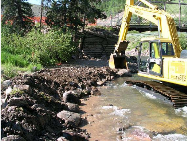
Photo 3. During construction, placement of large boulders to stabilize banks ( d_{50} calculated by hydraulic engineer)
